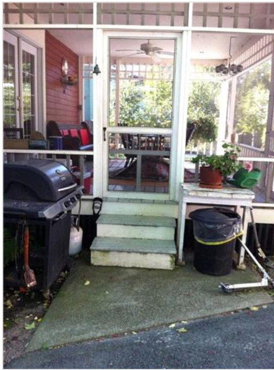
REC railing missing at back entrance
