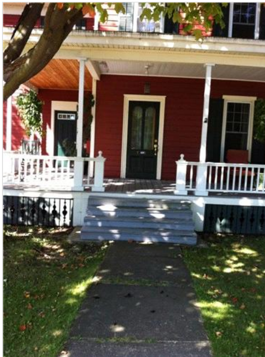
REC missing railing at front steps
