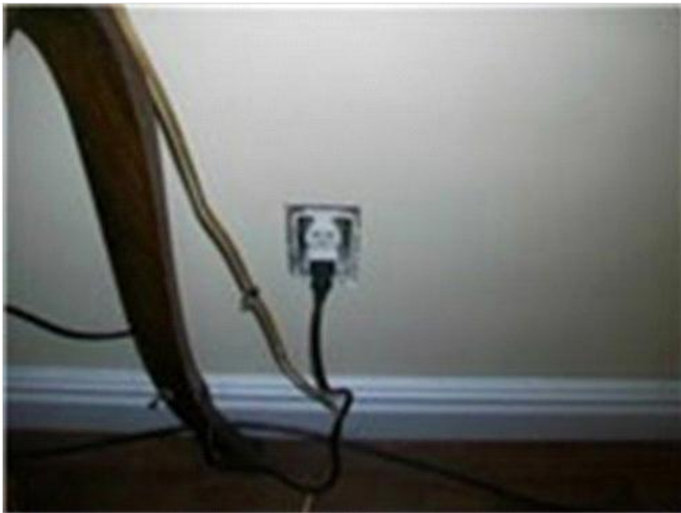
REC missing outlet cover in diningroom
