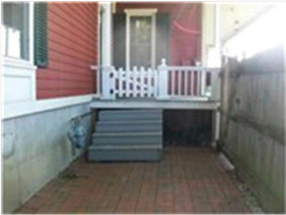
REC uneven steps and missing railing at side steps
