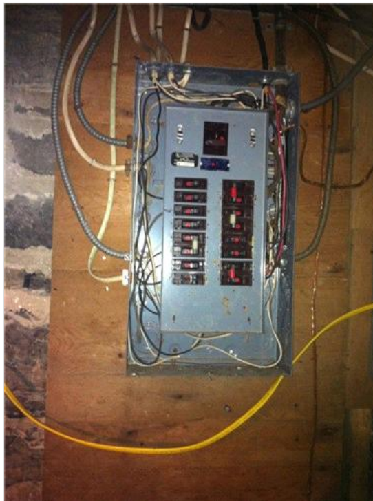
REC missing cover and loose wire should be restapled
