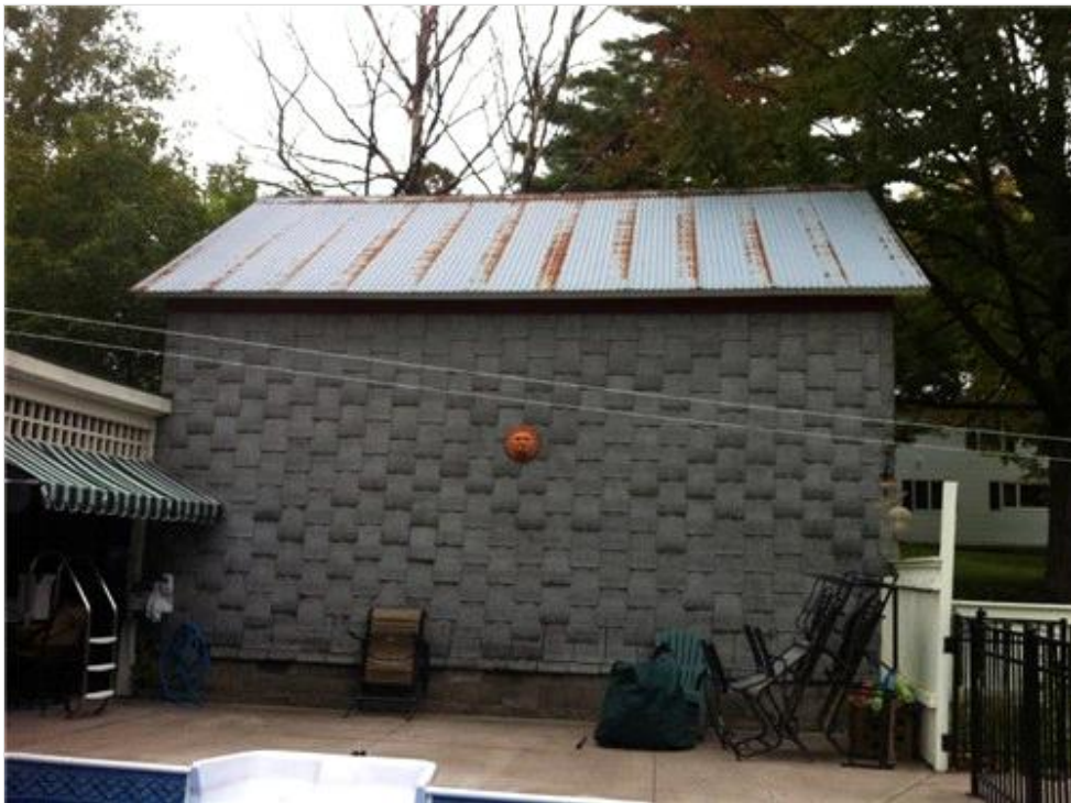
REC rusted roof on garage
