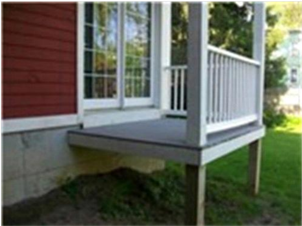
REC missing steps
